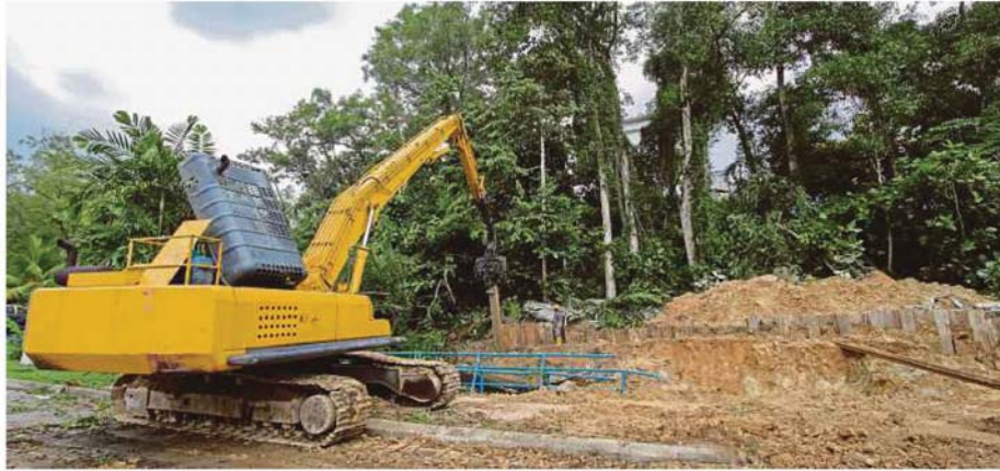
Repair work being carried out at the Taman Kelab Ukay 4 residential area in Bukit Antarabangsa, Selangor, yesterday. PIC BY AIZUDDIN SAAD
